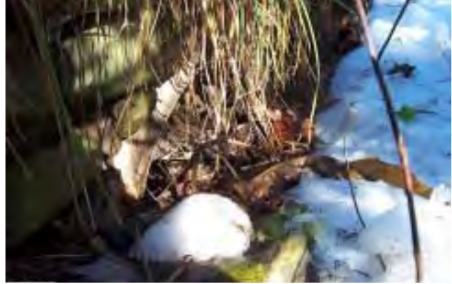
Photo 4. Corrugated metal culvert, right bank, stream out of the frame to the right.
