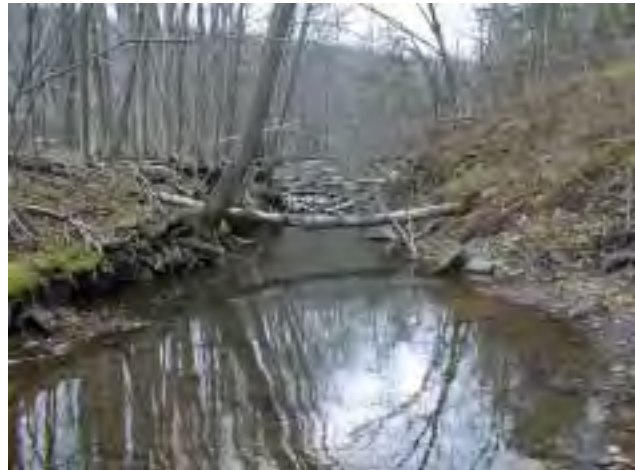
Photo 3. Looking upstream at eroding bank at monitoring cross-section 18, slumping clay bank at right, undercut trees at left.
