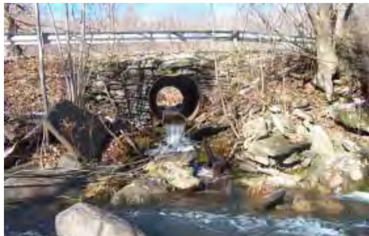
Photo 2. Four-foot diameter culvert, providing a crossing over Broadstreet Hollow Road for a major tributary to the main Broadstreet Hollow Stream. Flow in the main stream is from right to left.
