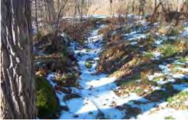
Photo 3. Culvert outlet swale on floodplain, right bank, Broadstreet Hollow stream is behind the viewer, flowing right to left.
