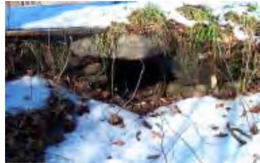
Photo 4. Close-up view of culvert outlet under Broadstreet Hollow Road (see also Photo 3).
