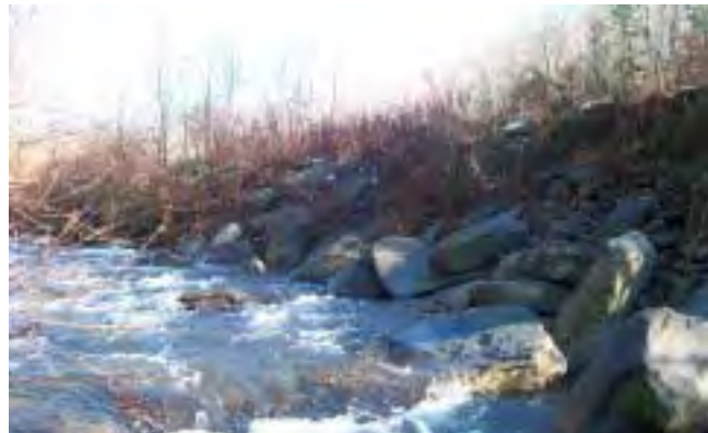
Photo 5. Looking upstream at slumping riprap on left bank of MU 7.
