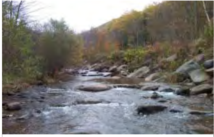
Photo 10. Looking upstream at native boulder rip-rap on left bank at the bottom of MU7. Note dense native riparian vegetation on the opposite bank, and sparse vegetation all along the rip-rap bank.
