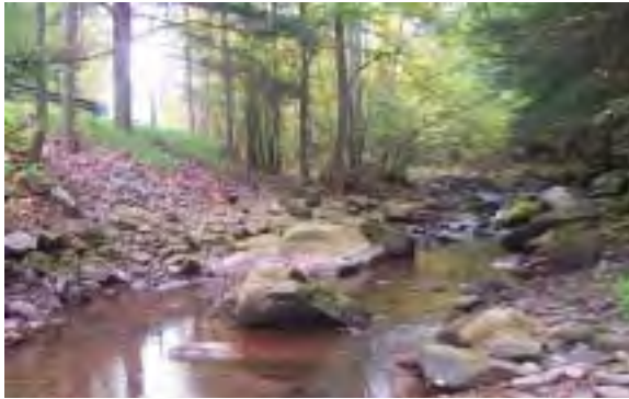
Photo 7. Looking upstream into the top of MU10, dumped rock fill at left in foreground, bank run gravel material at left in background, Broadstreet Hollow Road at top of bank.
