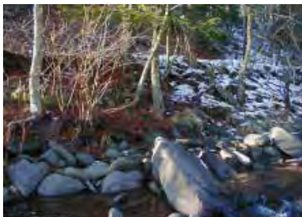
Photo 14. Right bank along Broadstreet Hollow Road embankment, showing steep slope, leaning trees and active stream processes at the toe (base) of the bank. Stream flow from right to left.
