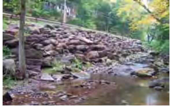
Photo 4. Looking upstream at stacked rock wall along road embankment, installed 2002 by Town of Shandaken Highway Department.
