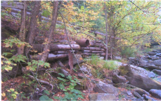
Photo 11. Looking upstream toward smooth metal culvert in log crib wall on right bank, along Broadstreet Hollow Road embankment. Culvert was dry at the time of the 2001 stream survey.
