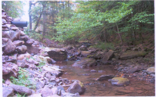
Photo 8. Looking upstream, black plastic corrugated culvert in stacked rock wall at left, draining inboard roadside ditch on Broadstreet Hollow Road.
