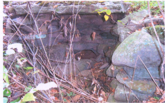
Photo 12. Culvert providing drainage for private road, on the left bank opposite and parallel to Broadstreet Hollow Road. Stream is behind the viewer, flow from left to right.
