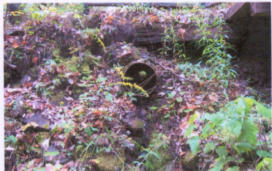
Photo 10. Smooth metal culvert on right bank, draining inboard ditch on Broadstreet Hollow Road, just downstream of private bridge crossing. Stream is behind the viewer, flow from right to left.
