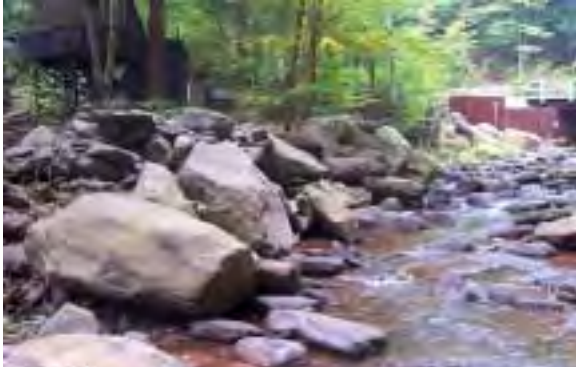
Photo 13. Looking upstream at right bank boulder berm, just downstream from County Bridge 3-34671-0.
