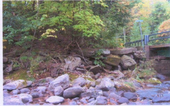
Photo 6. Large boulder rip-rap on left bank, just upstream from the David Merwin bridge. Stream flow is from left to right. Note partially stacked structure increases rip-rap stability.
