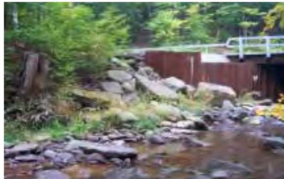
Photo 9. Looking upstream toward rip-rap and sheetpiling (bridge wing wall) along downstream from County Bridge #3346710. Stream flow is from right to left.
