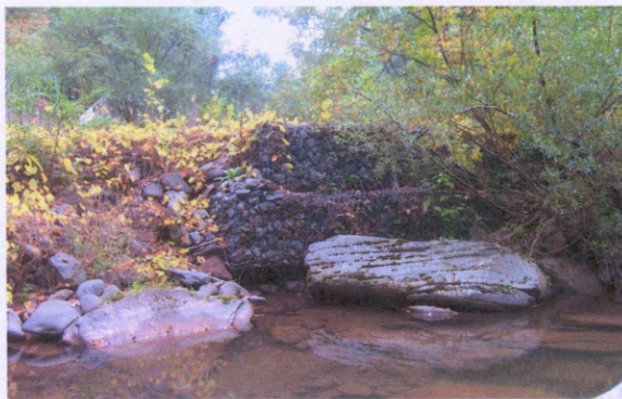
Photo 7. Gabion basket stream bank revetment, with willows upstream on right bank just downstream from the David Merwin Bridge, with minor "eddy erosion" on the downstream edge. Stream flow is from right to left.
