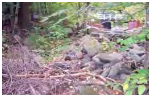
Photo 14. Back side of boulder/debris berm at 108 Broadstreet Hollow Road property, stream to the right.
