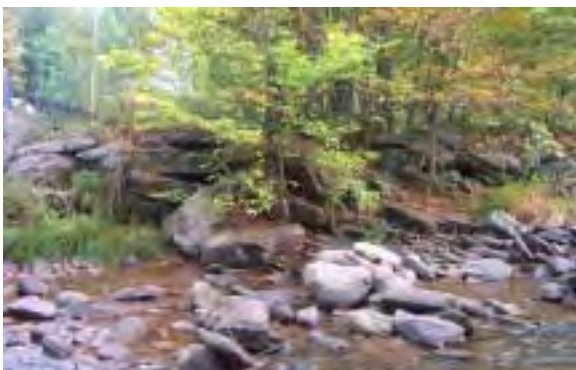
Photo 5. Boulder rip-rap on the right bank, just upstream from the David Merwin bridge. Stream flow is from right to left.
