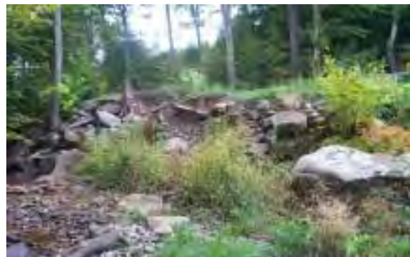
Photo 16. Left bank rip-rap and road fill erosion, upstream from County Bridge 3-34671-0, Broadstreet Hollow Road at the top of the bank. Stream flow is from left to right.
