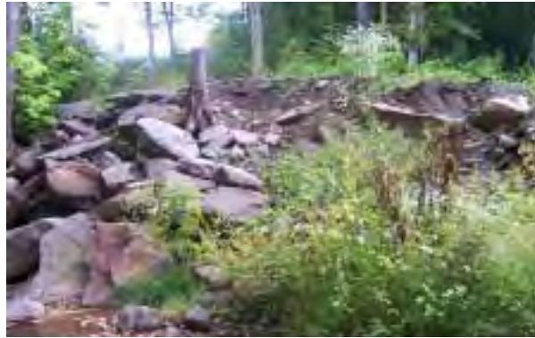
Photo 10. Partially failing rip-rap along left bank, just upstream of County Bridge 3-34671-0. Stream flow is from left to right.
