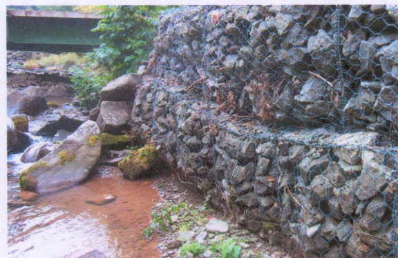
Photo 8. Looking upstream, gabions on left bank, downstream of David Merwin County Bridge 2-22457-0.
