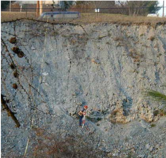
Photo 4. View of eroded left bank on DEP property. Material undercut and slumping.
