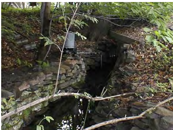
Photo 1. View looking upstream toward culvert under Mutton Hill Road. Laid-up stone walls on both banks, small pump on right bank.
