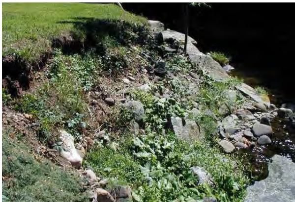
Photo 17. Dislodged riprap at left bank behind Town Hall parking lot-view looking downstream with dry hydrant partially visible in the background.
