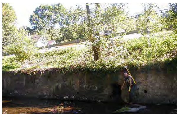
Photo 16. Concrete wall with box culvert along Route 55 between River Road and Fire House.
