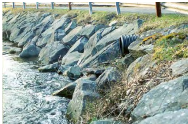
Photo 12. Looking downstream at rip rap along sharp curve and culvert on right bank, along River Road upstream of bridge. Flow hits directly into bank near culvert.
