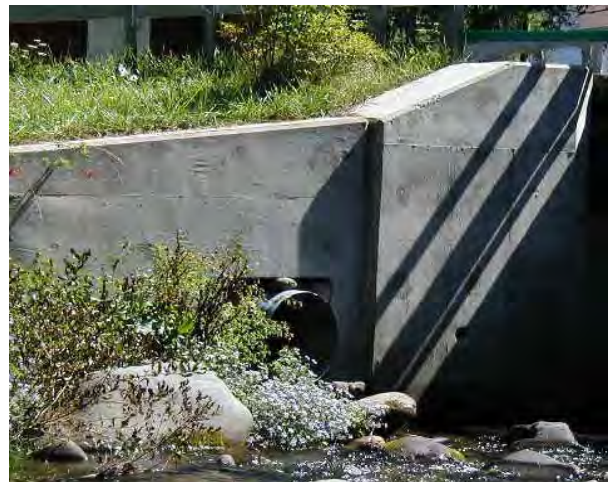
Photo 14. Culvert in left bank abutment on upstream side of River Road Bridge, view looking downstream from the center of the stream.
