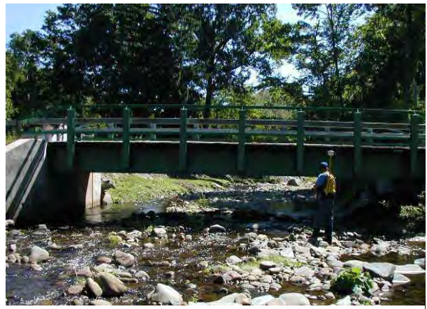
Photo 8. Looking downstream at River Road Bridge, just above Town Hall. Note the cobbles that are deposited upstream of the bridge in the foreground of the photo.
