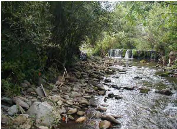
Photo 11. Looking upstream towards Davis Lane Bridge concrete grade control structure over sewer line.
