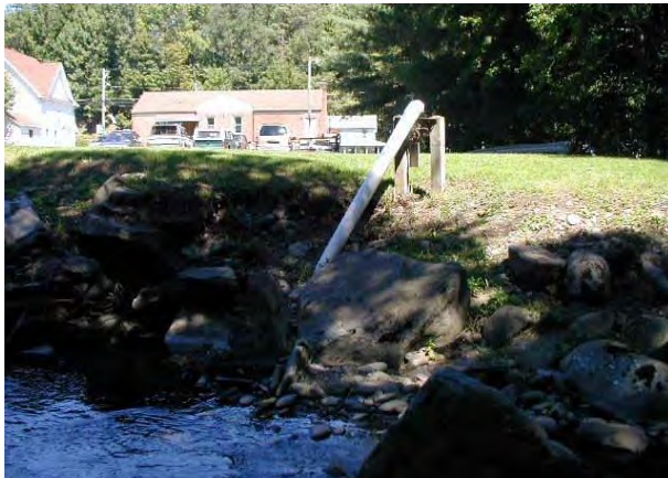
Photo 13. Dry hydrant (out of order, removed) and eroded bank behind Town Hall parking lot-view looking toward left bank & Town Hall from center of stream. (flow left to right)
