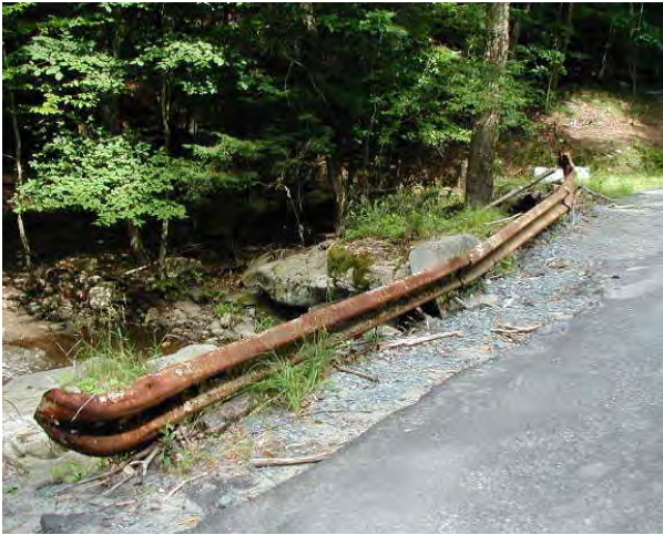
Photo 4. Recent storms have overtopped the road at this culvert, causing damage to the road. FEMA funding replaced guardrail seen in photo, 2002.
