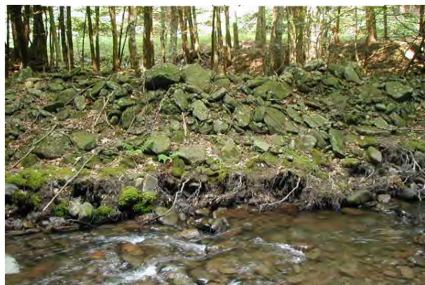
Photo 10. Looking at undercut right bank and berm, stream flow left to right.
