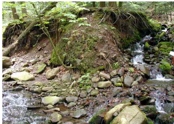
Photo 3. View looking upstream at left bank and confluence with another tributary downstream of Photo 2 (on right side of the photo) that flows under Camp Road. Significant erosion.
