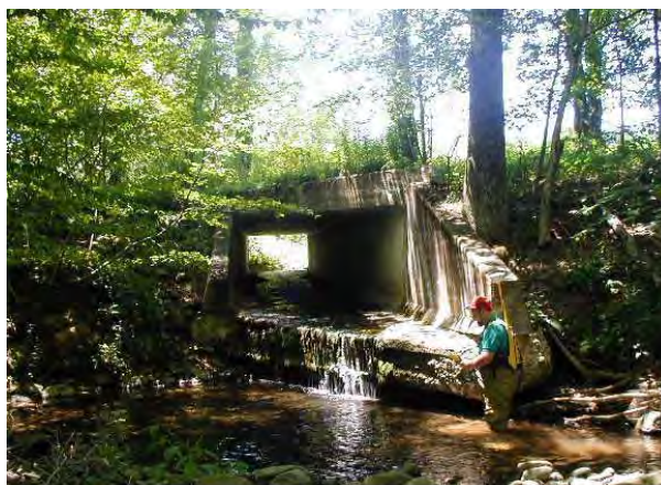
Photo 7. View from mid channel looking upstream. Scour pool at outlet of Route 42 box culvert. Eroding right bank 10' high.
