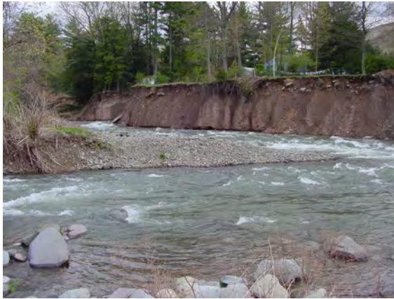
Figure 3. Streambank failure along project reach (May, 2002)
