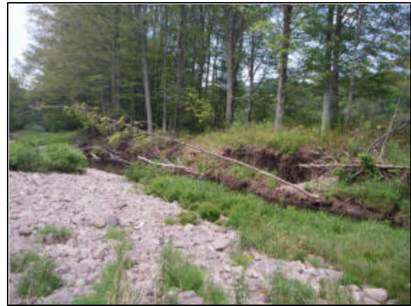
Erosion at Stations 43980 - 43791
