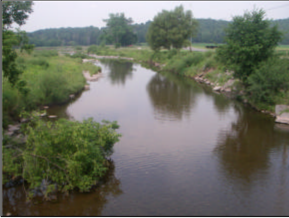
Rip-rap at Stations 40130 – 39983 Woody debris at Station 40095 Riparian planting sites at Station 39922
