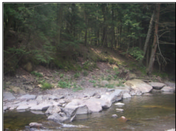
Erosion at Stations 37900 - 37857
