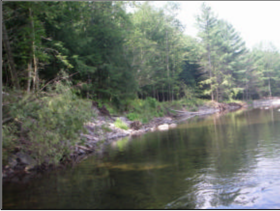
Erosion at Stations 25219 - 24929
