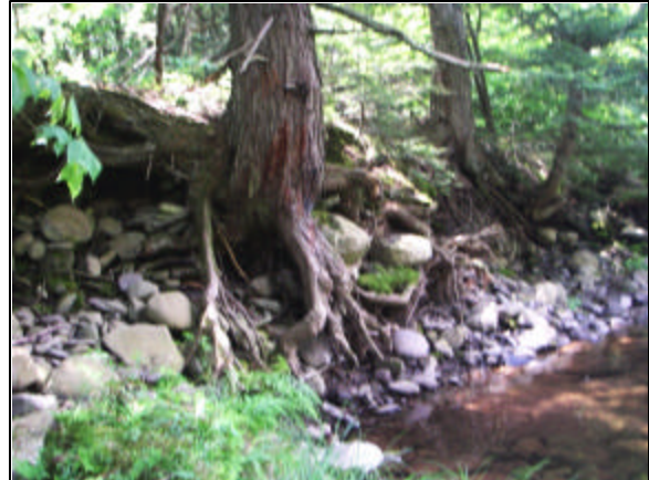
Erosion at Stations 15360 - 15319
