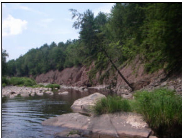
Mass failure and clay exposure at Stations 13961 – 13005
