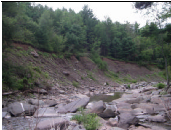
Erosion at Stations 4655 - 4013
