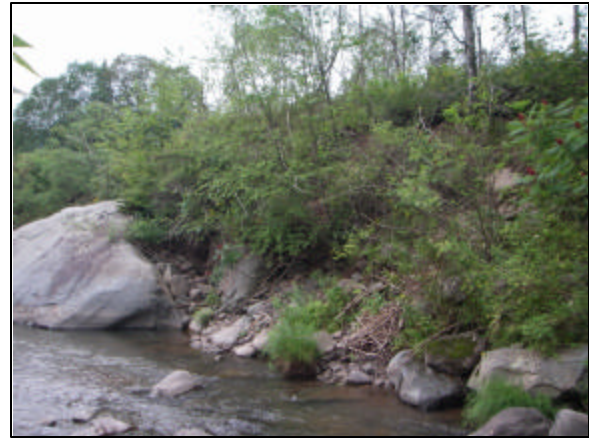
Erosion at Stations 4991 - 4788
