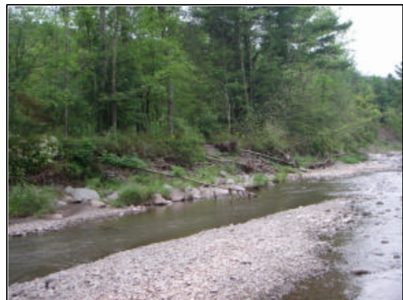
Erosion at Stations 5188 - 4925
