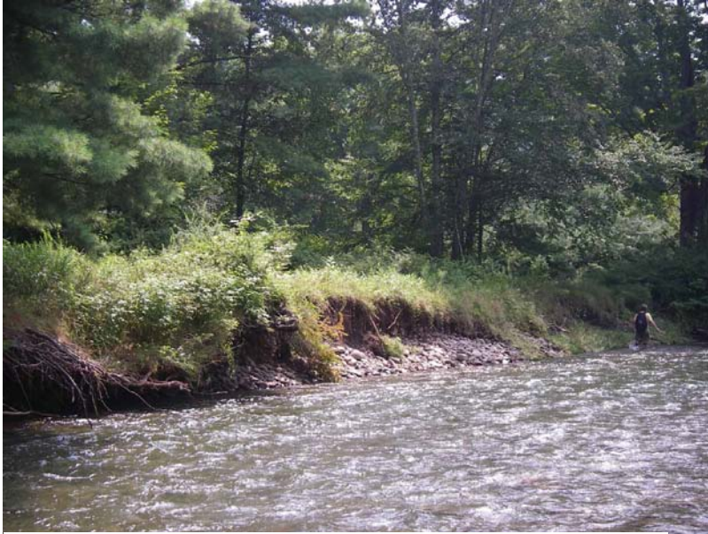
Figure 10 Bank erosion adjacent to a mowed field along the left bank
