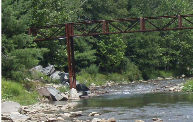
Figure 15 Rip-rap and erosion at right pier of footbridge
