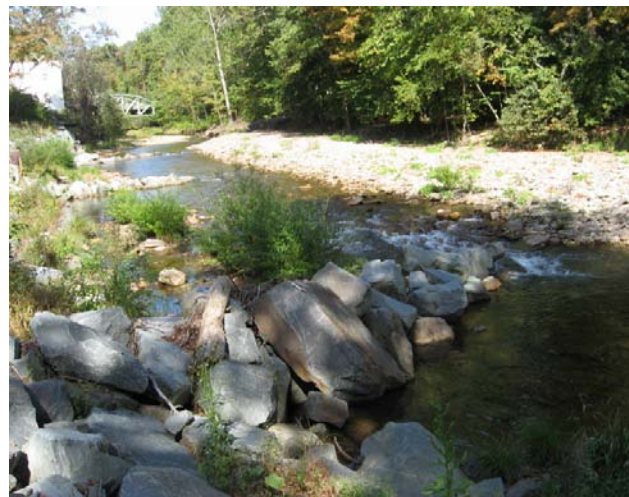
Figure 8 Looking upstream. Barbs installed to deflect flows away from the right bank
