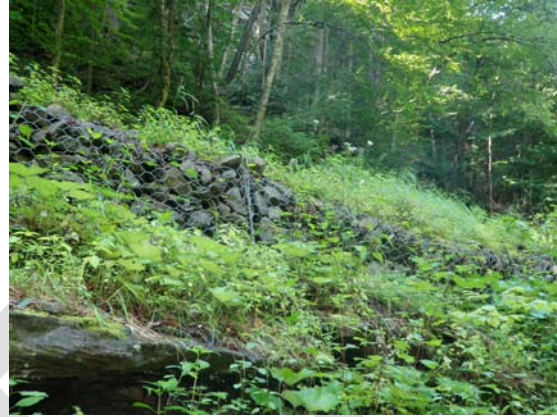
Figure 7 Compromised gabion basket revetment
