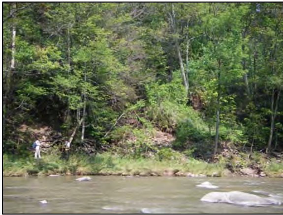
Bank erosion at Station 32900
