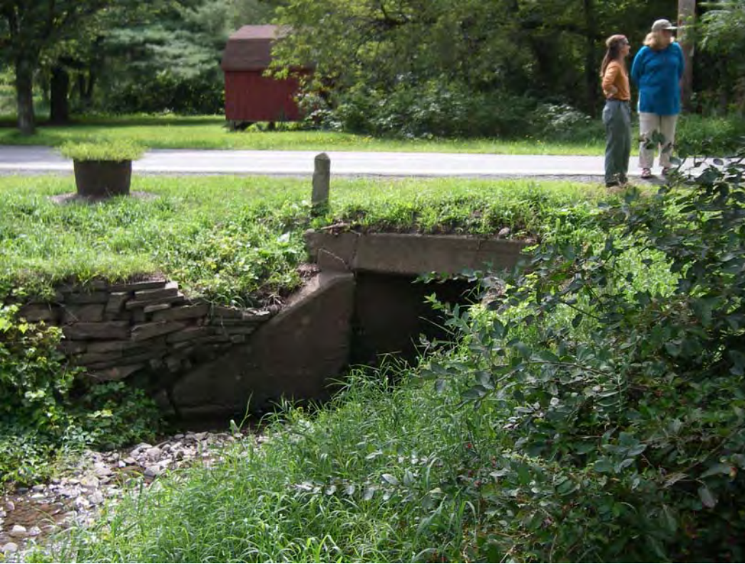
Photo 1: View looking downstream at entrance to existing concrete culvert. Note failed headwall.
