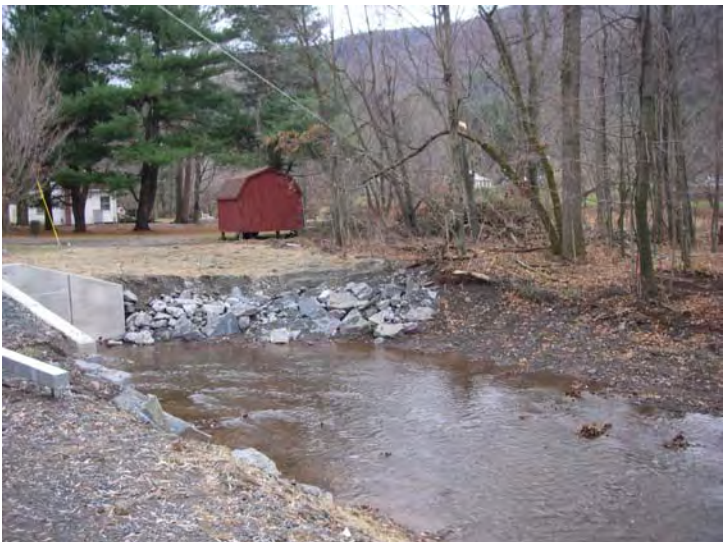
Photo 13: Culvert outfall and small rock on left bank. Trees, shrubs and willows were planted for long term stability
