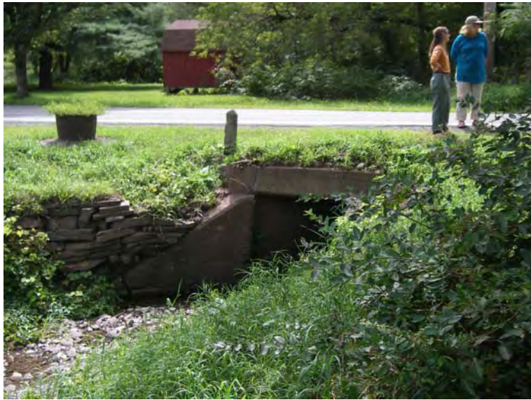
County Route 13A Culvert to be replaced
