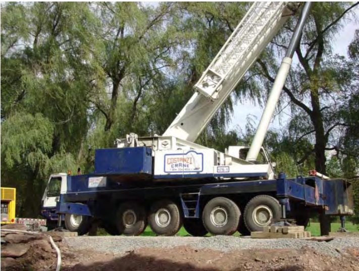
Photo 9: A large crane was needed to lift and set sections, power lines needed to be relocated to facilitate setting of the sections.
