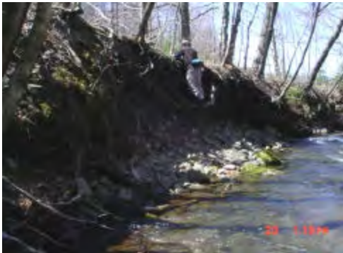
Bank Erosion, with narrow, undercut buffer
