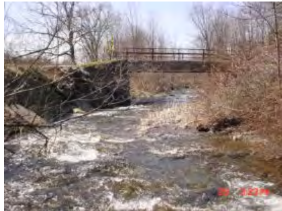
Spruceton Road Bridge, #3201250. Note loss of floodplain connectivity due to entrenchment at bridge
