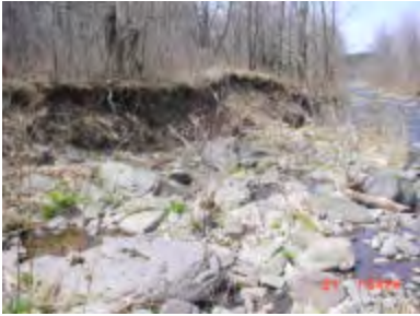
Bank Erosion, left
