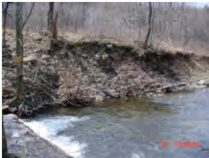
Bank Erosion, left (Inset F, Fig. 4.3.2)
