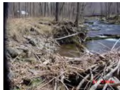
Bank Erosion, right
