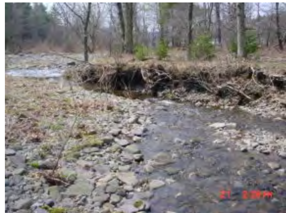
Bank scour near convergence
