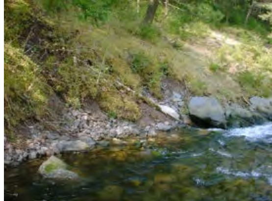
Toe protection only, small headcut at head of riprap
