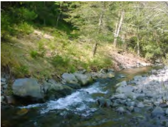
Erosion extending downstream of rip rap
