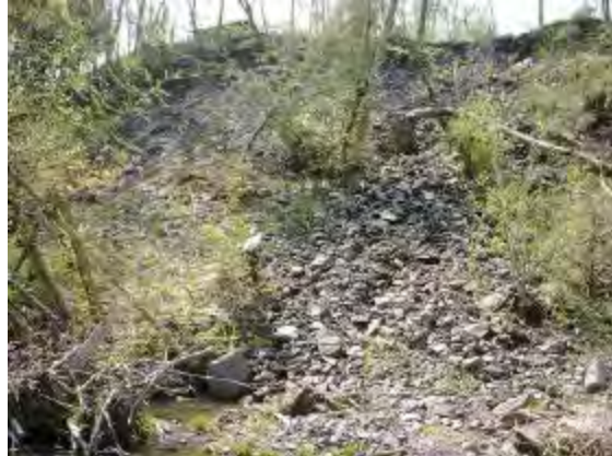
Large slope failure
