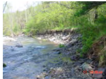
Bank Erosion, right bank
