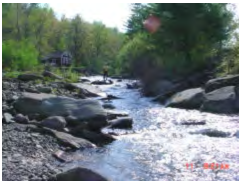
Headcut at divergence of overflow channel and debris jam
