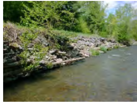
Dumped rip-rap over failing crib wall
