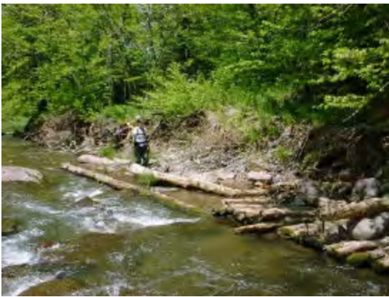
Erosion at downstream end of crib wall
