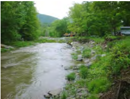
Bank erosion, right
