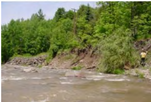
Bank erosion, right
