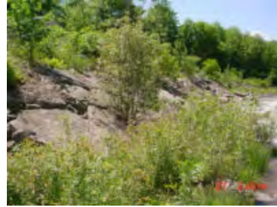
Rip Rap, left
