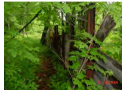
Flash Boards, left
