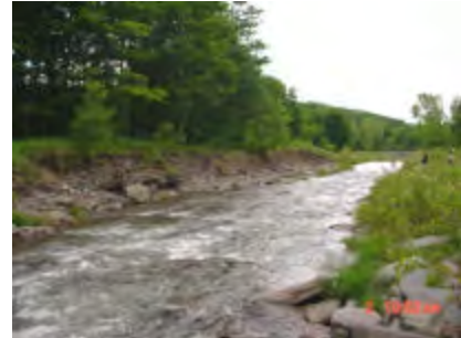
Bank erosion, left
