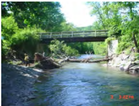
Debris Jam on approach to bridge
