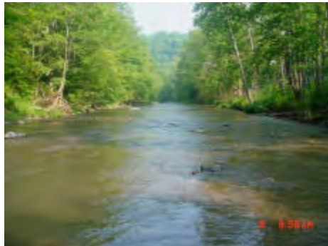
Aggradation downstream of bridge
