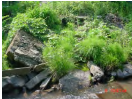
Culvert outfall over dumped riprap
