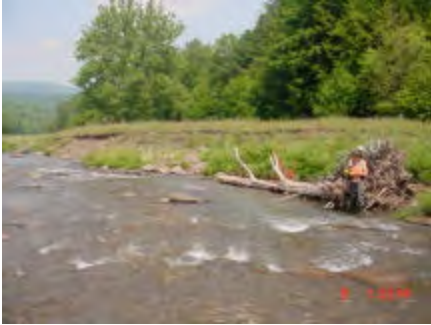
Bank erosion on alluvial terrace, right
