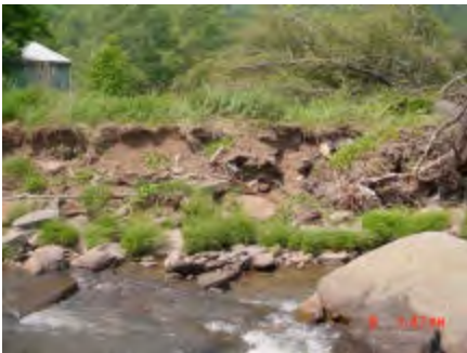
Dump site exposed by erosion, left
