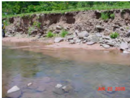
Worsening streambank erosion in 2005
