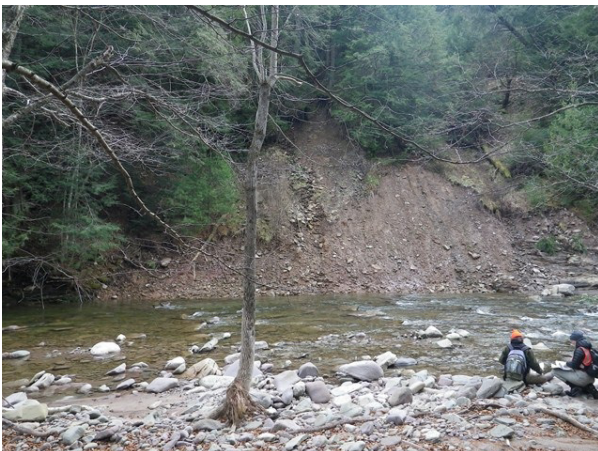
Slope failure on the left bank. (IMG1603)
