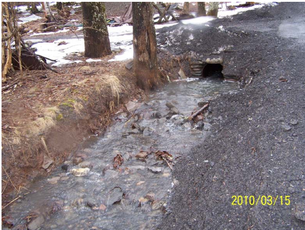
Figure 5 Example of street runoff and bank erosion in ditch 2
