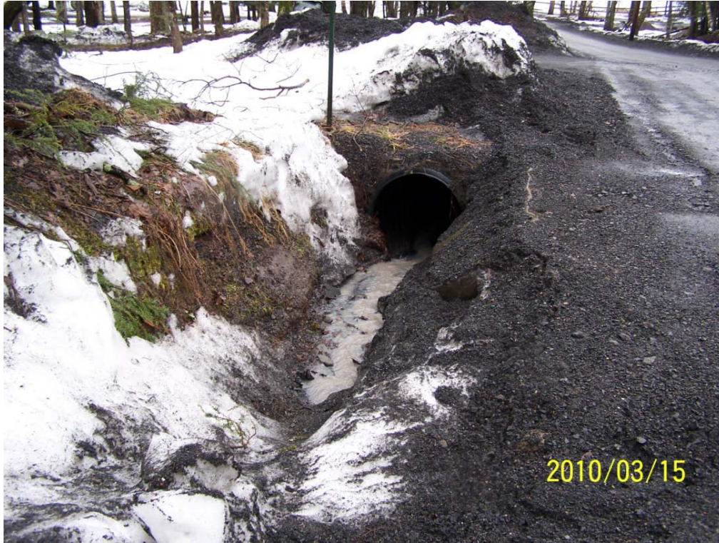
Figure 4 Example of street runoff and bank erosion in ditch
