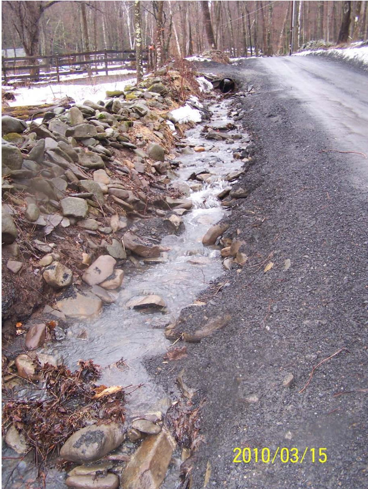
Figure 6 Example of street runoff and bank erosion in ditch 3
