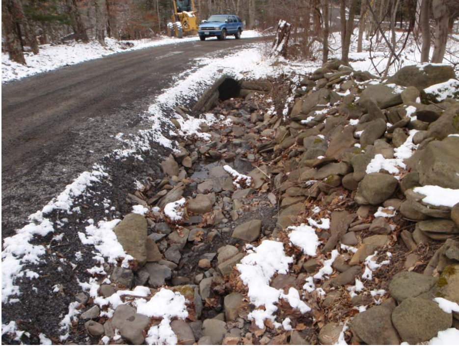
Figure 2 Example of eroding banks adjacent to Cross Patch Road.
