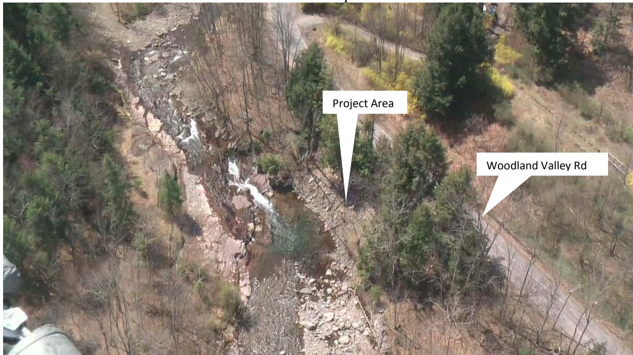
Figure 1 Top photo shows undercut road at the top of the failing bank. Bottom photo is an aerial photo of Woodland Valley Creek, project location and proximity to the road.
