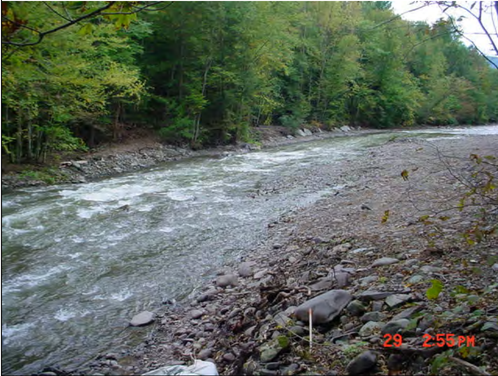
Figure 1: top of project are looking down stream. This section has been completed and is scheduled for bio engineering this fall.
