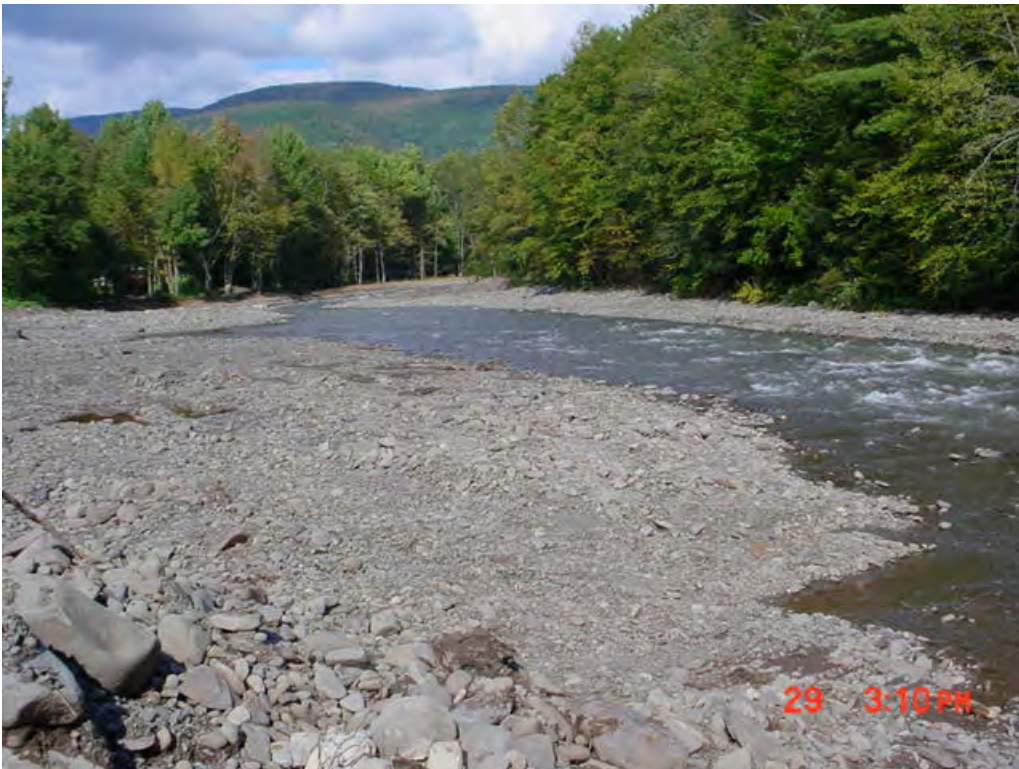
Figure 4: Looking upstream from near station 14+00. this section is incomplete, and scheduled for temporary seeding and mulching.
