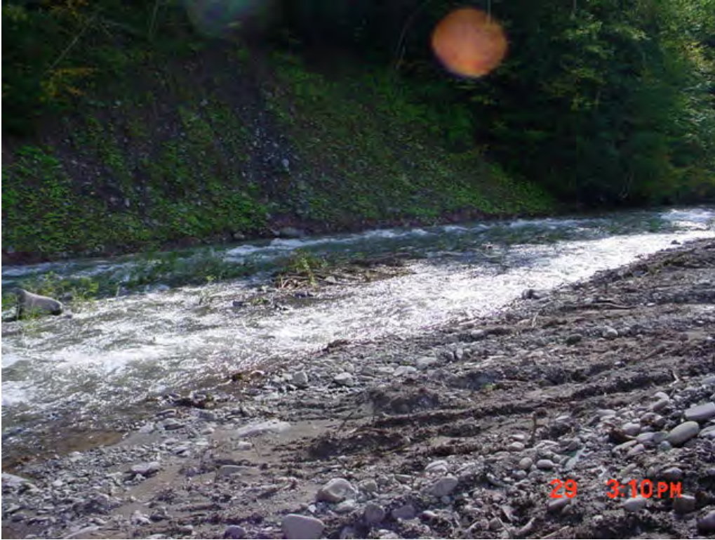
Figure 5: Problem bank near bottom of project area. This section has not been completed. Temporary flood conveyance has been provided on the opposite bank to relieve stress on the problem bank. This area will be treated with temporary seed and mulch.
