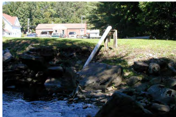
Photo 3. Dry hydrant behind Town Hall parking lot. View looking toward left bank from center of stream.
