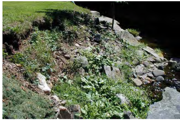
Photo 1. Erosion – left bank behind Town Hall. View looking downstream, dislodged riprap visible in right front corner of photo.
