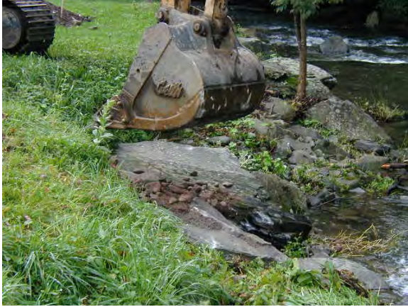
Photo 4. Dislodged riprap removed from the creek and keyed into the eroded bank to create a bankfull bench on September 26, 2003.
