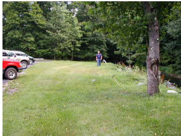
Photo 2. Top of bank before construction. Damaged Black Cherry on right, dry hydrant shown in the distance; both were removed.
