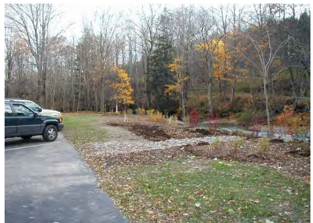
Photo 7. View looking downstream from parking lot. Shows completed swale and planted buffer.
