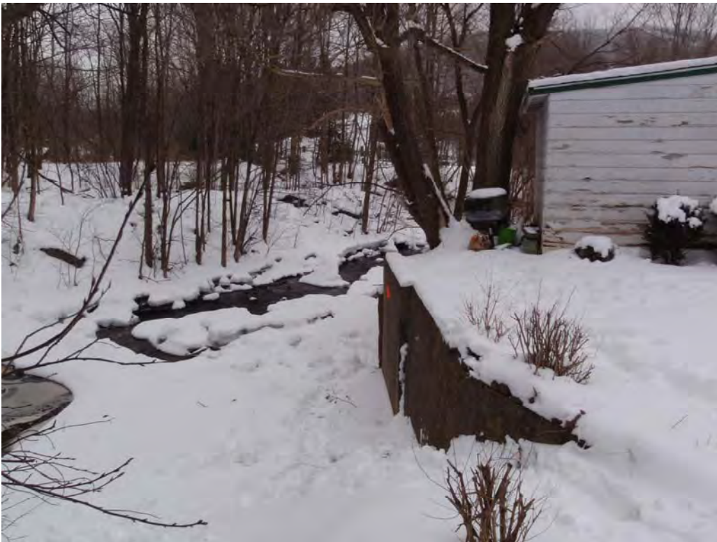
Downstream view showing cracked retaining wall, 2010
