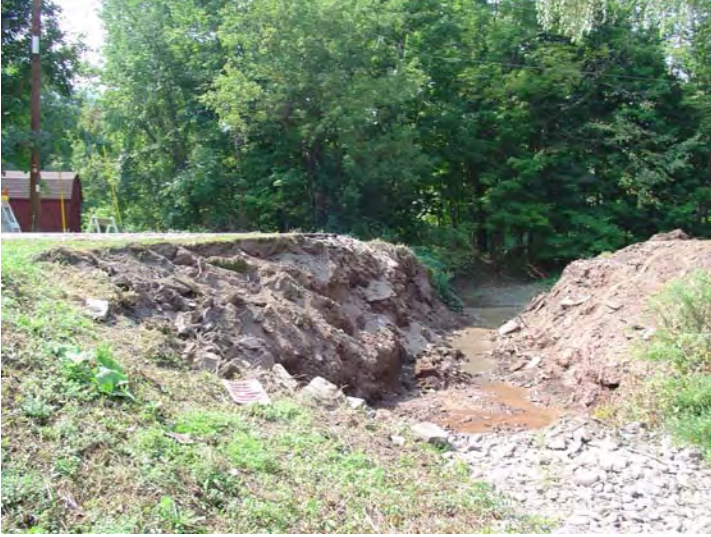
Photo 5: Old culvert removed and ready for excavation and preparation of the culvert base.
