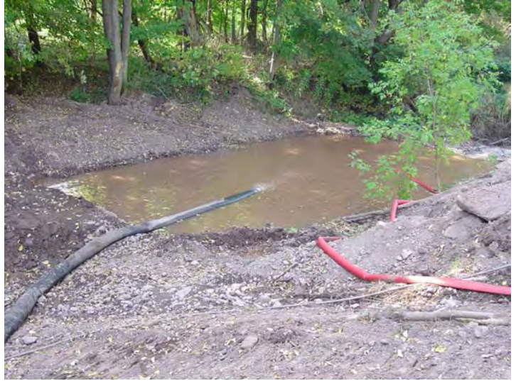
Photo 6: Temporary settling basin constructed in the down-stream channel to treat sediment laden water.
