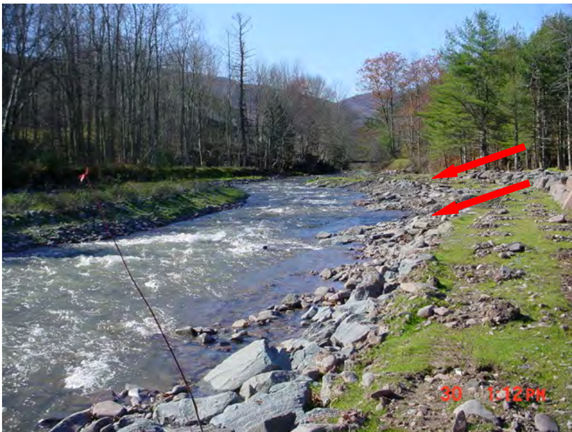
Figure E6 Two rock vanes (red arrows) on lower third of right bankfull bench. Note that turbulent flow is moved off-bank, toward center of channel. Bench is seeded and planted with potted material.
