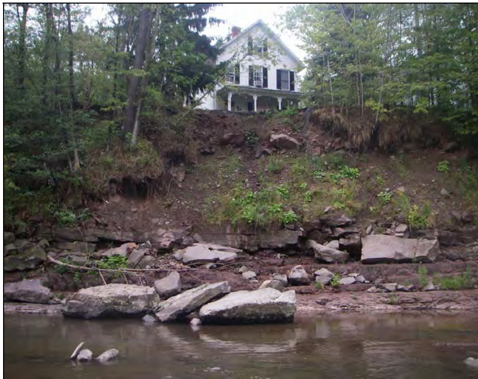
Figure 1 - Bank Failure at Schoharie Street Project Site
