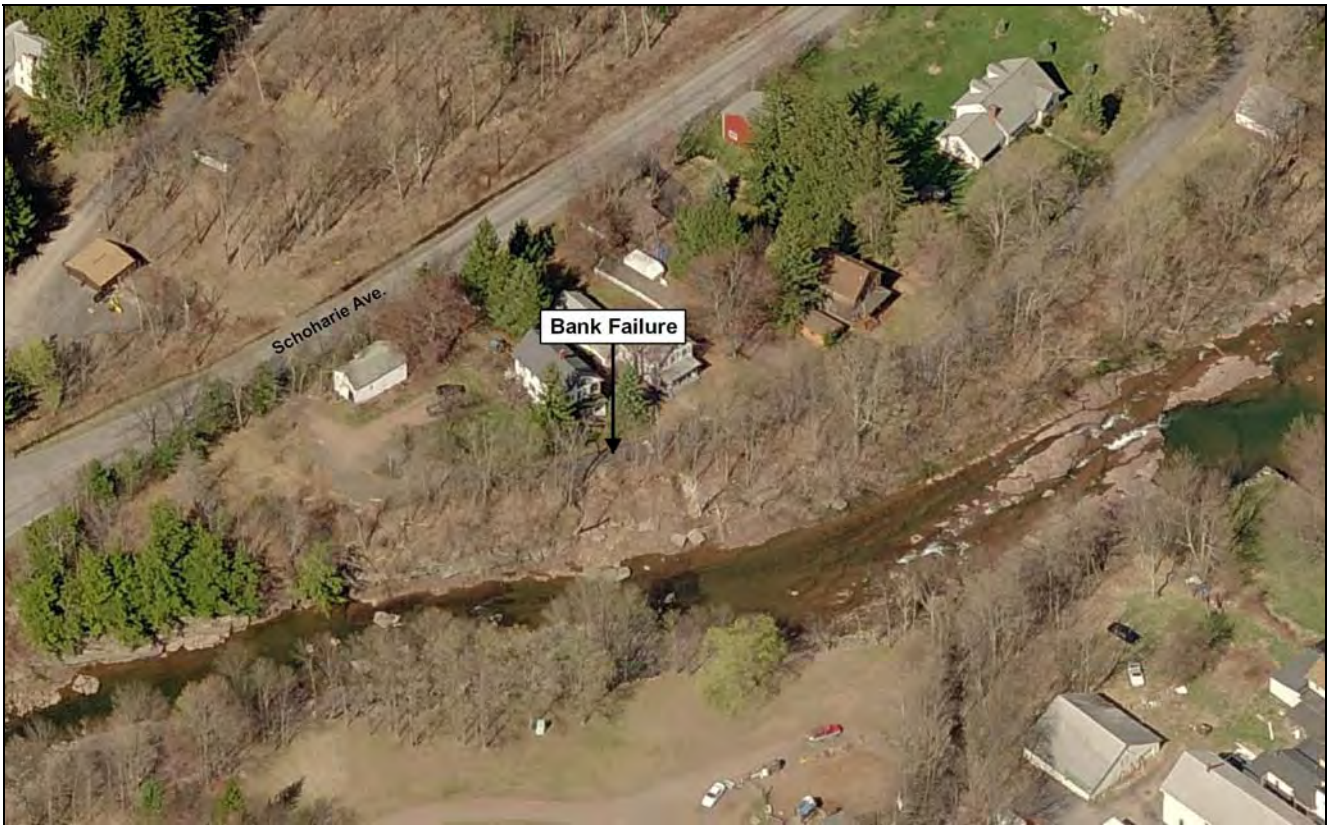
Figure 2 - 2006 aerial photograph of bank failure at Schoharie Street Stabilization Project
