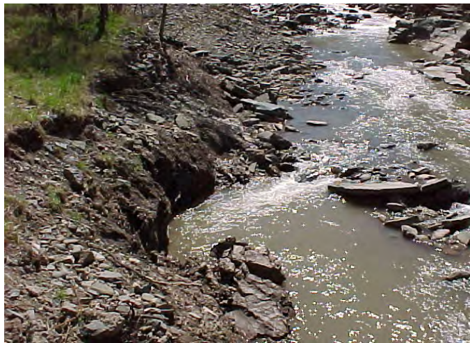
Figure 1: Extensive clay exposures due to channel down cutting presented a significant water quality impact, as well as extensive infrastructure damage.
