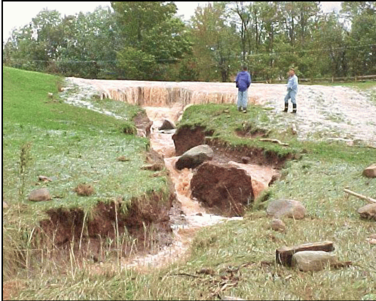
Figure IV-47: Damage to north emergency spillway on the C.D.Lane dam as the result of flows from tropical storm Floyd.
