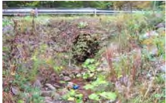
Photo 3. Looking upstream into tributary culvert under Broadstreet Hollow Road. Stream flow in the main channel (behind viewer) is from right to left.
