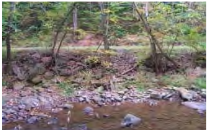
Photo 7. Dumped rock fill, along road fill/embankment on right bank, MU9 Stream flow is from right to left
