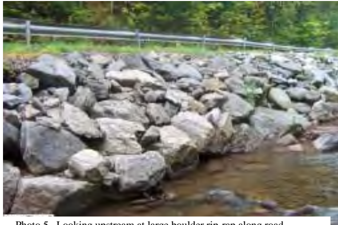
Photo 5. Looking upstream at large boulder rip-rap along road embankment, constructed following January 1996 flood.
