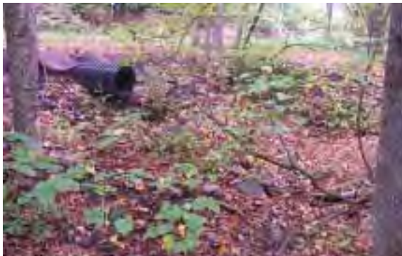
Photo 4. New culvert, right bank, MU9 – road above, Broadstreet Hollow stream behind and to the right of the viewer.
