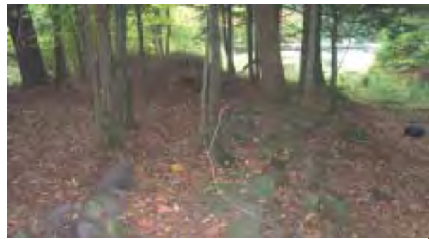
Photo 5. 295-foot earthen/cobble berm on the right stream bank, forming an embankment for the small pond. Pond is visible in the background to the right, stream is out of the frame to the left.
