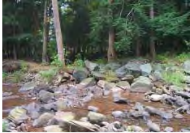
Photo 2. Right bank quarried boulder rip-rap, stabilizing pond inlet area. Note sycamore tree, being undercut at the roots. Stream flow is from right to left.
