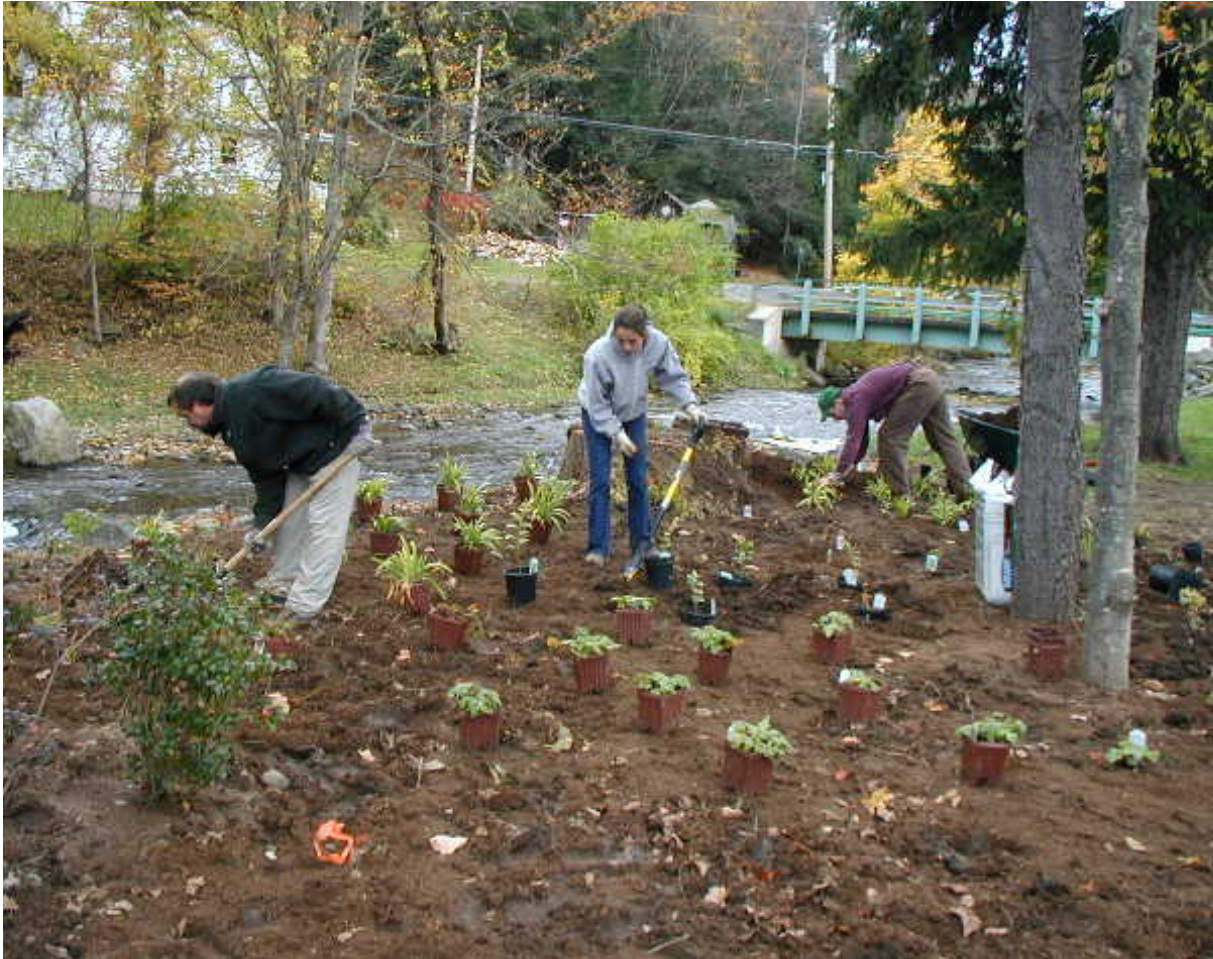
Town Hall Stream Restoration Demonstration Project. Photo taken by Lori Kerrigan, SCSWCD.
