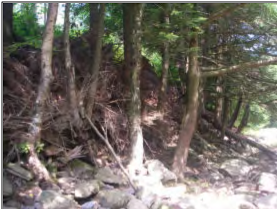
Erosion at Stations 63672 - 63516
